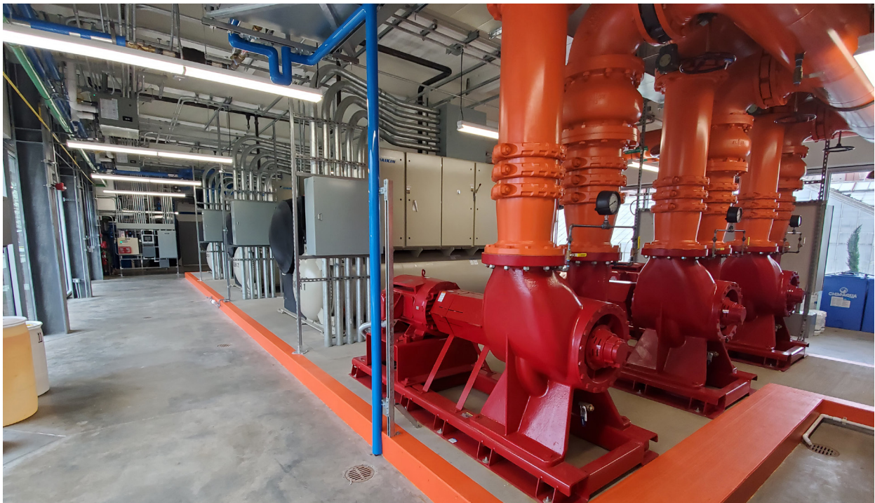
Oregon State University North District Utility Plant, Corvallis, Oregon
